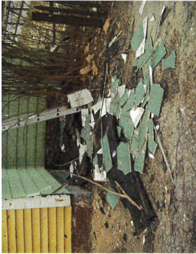
Improperly removed asbestos from home renovation project.
