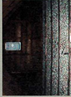
Vermiculite insulation found in an attic.
