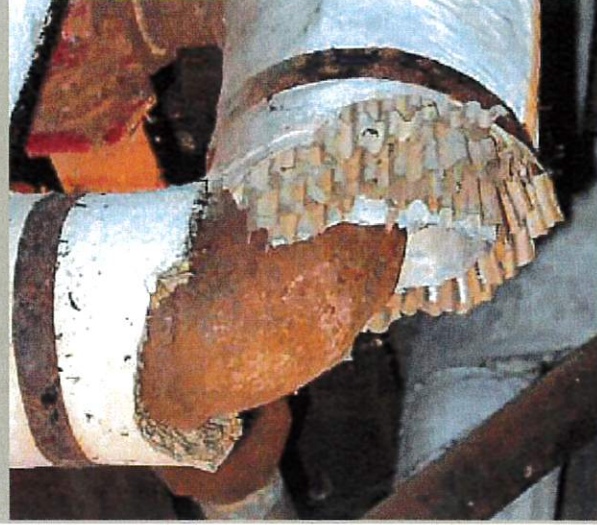
Damaged asbestos pipe insulation.
